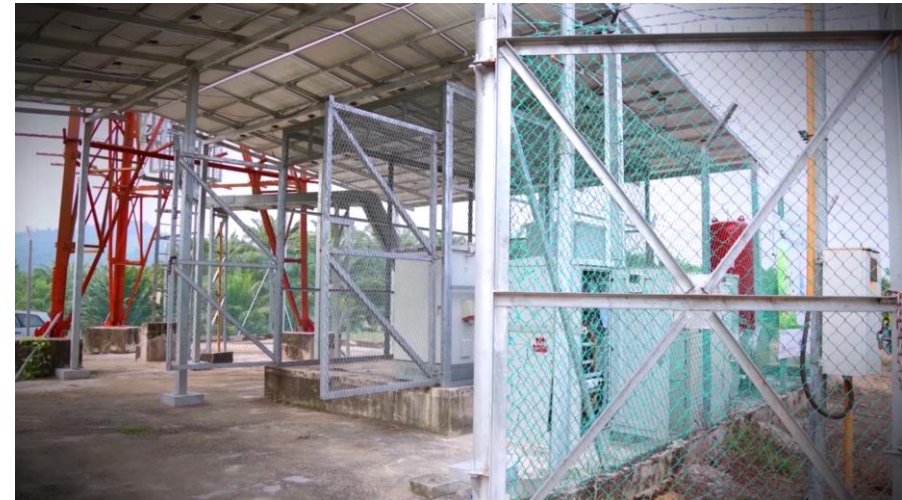
Energy storage for telecommunication tower in Malaysia
